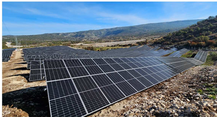
Fig. 26. Solar power plant "Solar Čevo"
